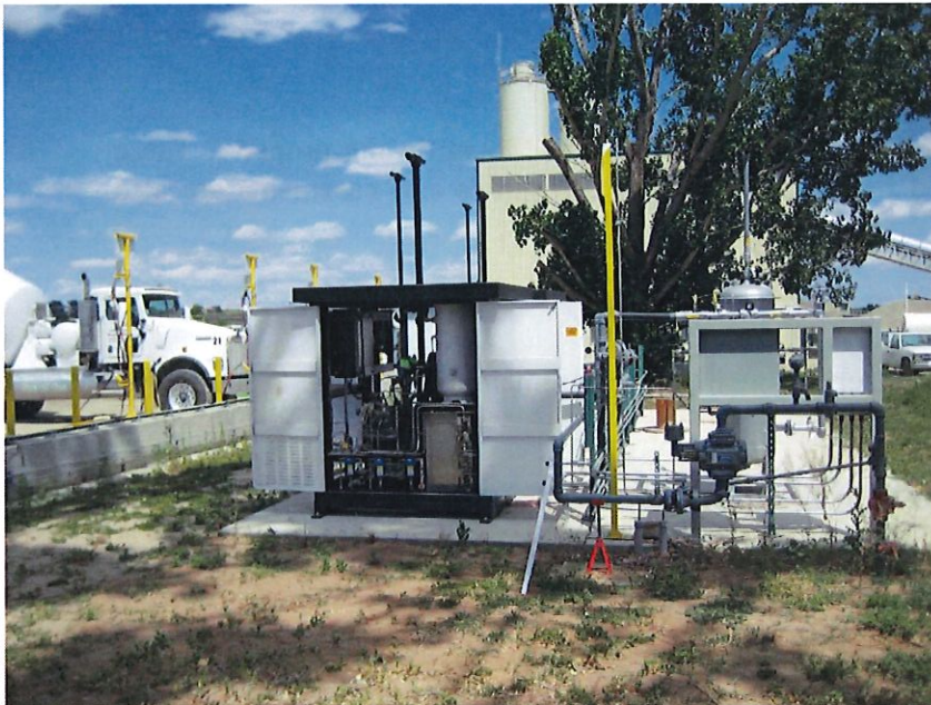
Photograph 2. Compressed natural gas station and fueling area.
